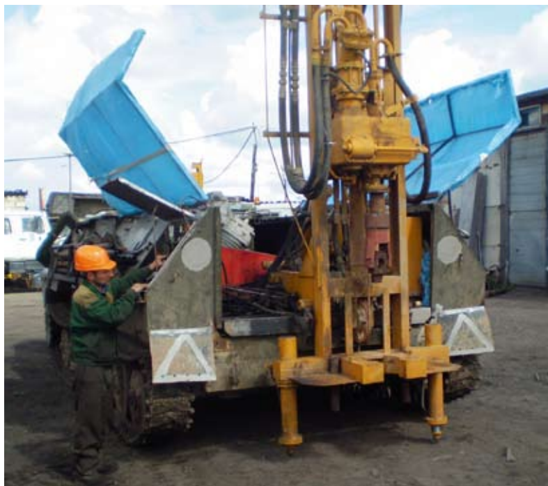
Drilling rig URB 2-A-2 based on a crawler cross-country vehicle MTLBU
